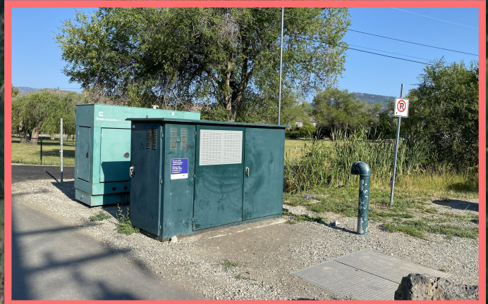
Woodsdale LS & Generator
