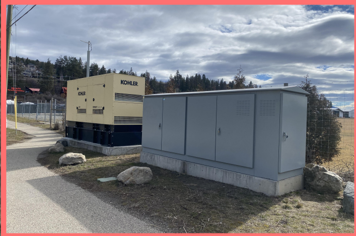
Lodge Road LS and Generator
