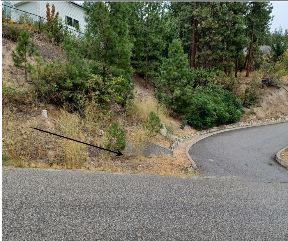
Photo 7: Looking upslope (northwest) from Forest Hills Dr towards property and mapped drainage hazard area. Location of two manholes at arrow. (August 9, 2023).
