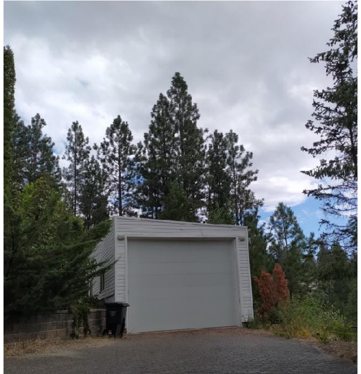
Front (north) side of existing structure to be replaced. Cedar hedge along the west side.
