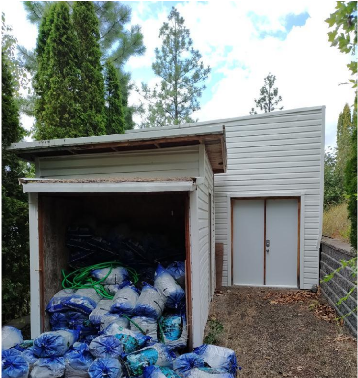
Backside of structure to be replaced. Hardscaped with debris accumulations (needles, litter etc).
