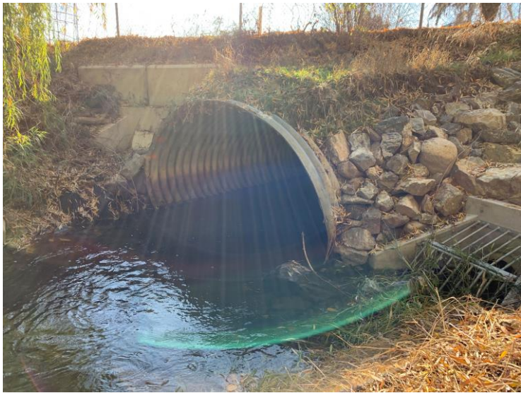
Woodsdale Road Outlet
