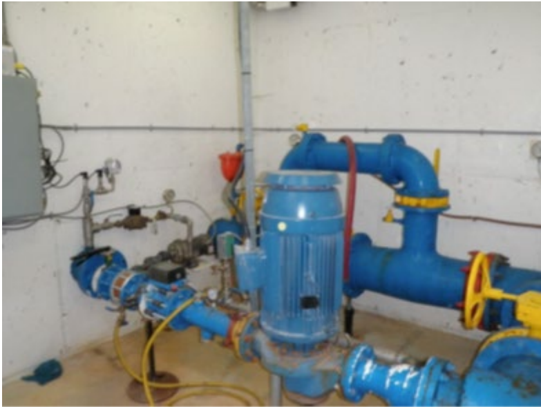
Picture of inside the existing Irvine Booster station
